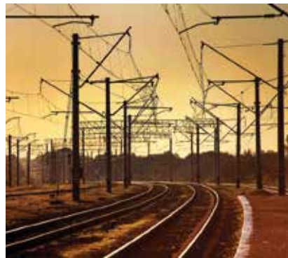
Railway signalling & pilot cables
